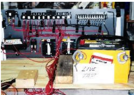
Live test of the electrical system on work bench using the vehicle battery.
